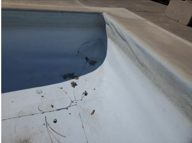
Photo 7: Wading pool liner failure
