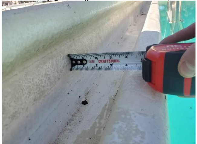
Photo 6: Dry gutters (pool shell movement)
