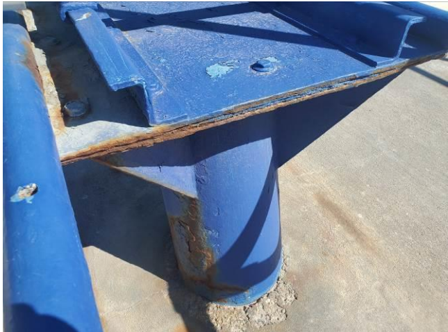
Photo 5: Corroded dive stands
