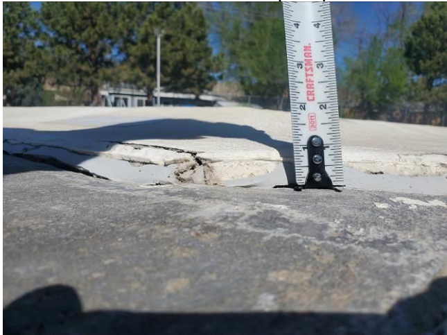
Photo 1: Toe stubbers around pool perimeter
